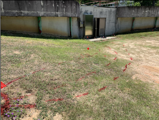
Electrical running toward electrical cabinet
