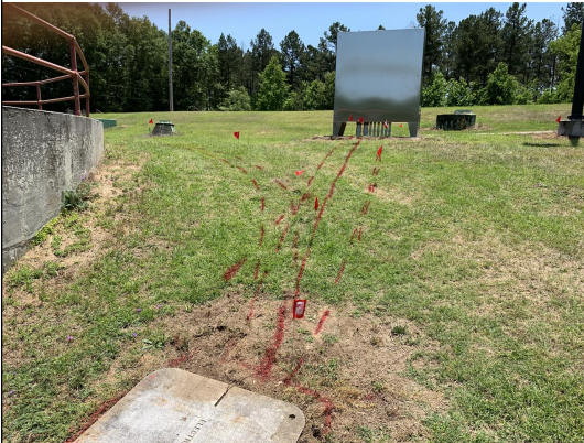
Several lines running into/out of electric vault
